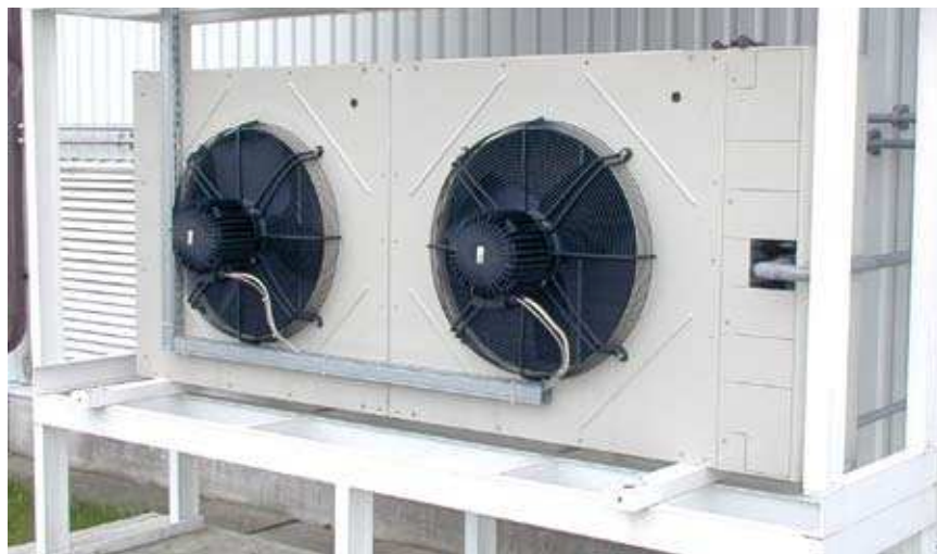
Cold storage infrastructure in China is more than seven million cubic meters
